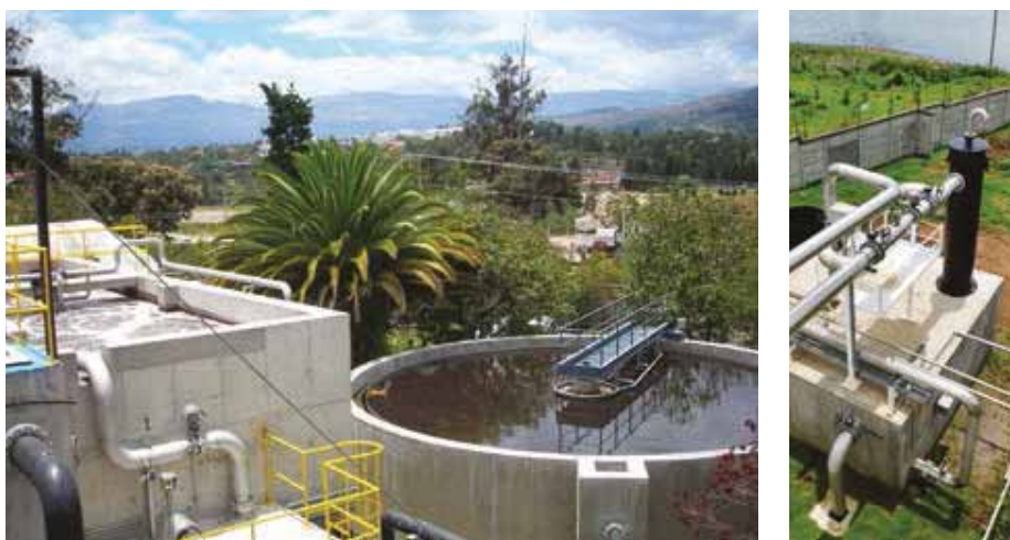
Left: Global Water Engineering’s anaerobic treatment plant is carefully integrated into the scenic landscape of Cumbaya, a suburb of Quito, Ecuador. Right: Carbon dioxide system installed at Compañía Cervecería de Nicaragua.
