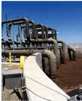
Six Mazzei model 12050 stainless steel injectors provide aeration for activated sludge digesters at the City of Atwater, California, Regional Wastewater Treatment Plant with a capacity of 42.4 million liters per day. Photo by Mazzei
